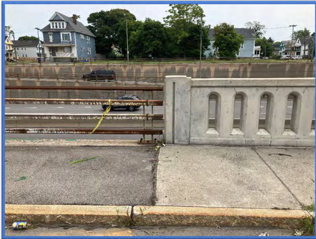
Photo 9 – Asbestos-containing railing post base caulk is associated with all of the metal guiderails located on top of the northern retaining walls. No asbestos-containing caulk is associated with the new decorative concrete guide rails located on top of the southern retaining walls.
