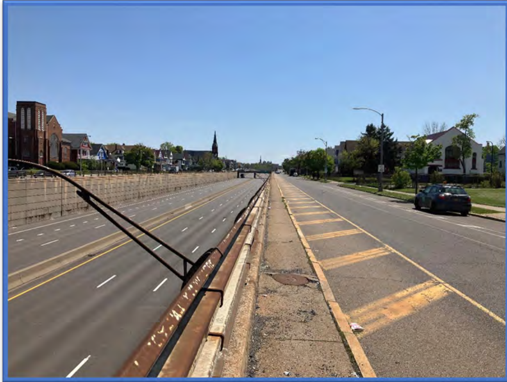
Photo 3 - View to the south from the southwest corner of the E Ferry Street Bridge over Kensington Expressway (Route 33) (BIN 1022640), with the highway retaining walls and East Utica Street over Kensington Expressway Bridge (BIN 1022630) visible in the background.
