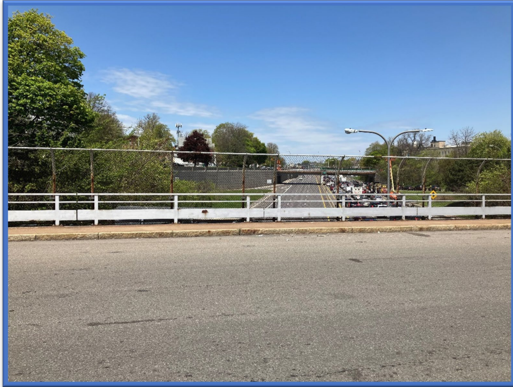
Photo 1 - View to the north from the middle of the E Utica St Bridge over Kensington Expressway (Route 33) (BIN 1022630).
