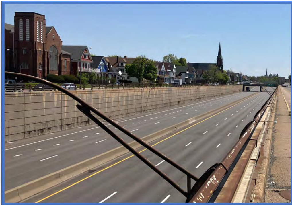
Photo 9 - Retaining wall system within the Kensington Expressway project corridor that has an associated asbestos-containing caulking located within each expansion joint and an inaccessible/assumed asbestos-containing waterproofing located on the back sides of the abutments, retaining walls, counterforts, and tops of footer piles.
