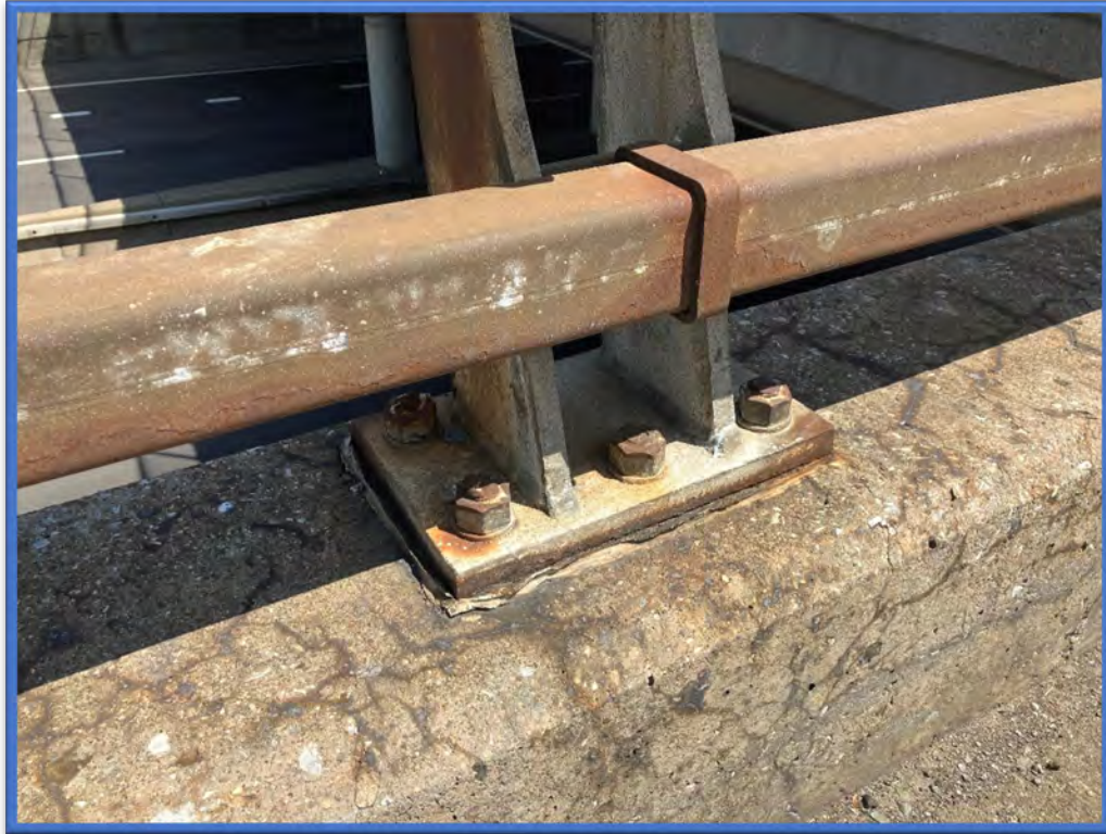
Photo 5 – Asbestos-containing railing post base caulk located at the top of the retaining walls near BIN 1022640. This ACM is present throughout the northern portion of the project corridor.
