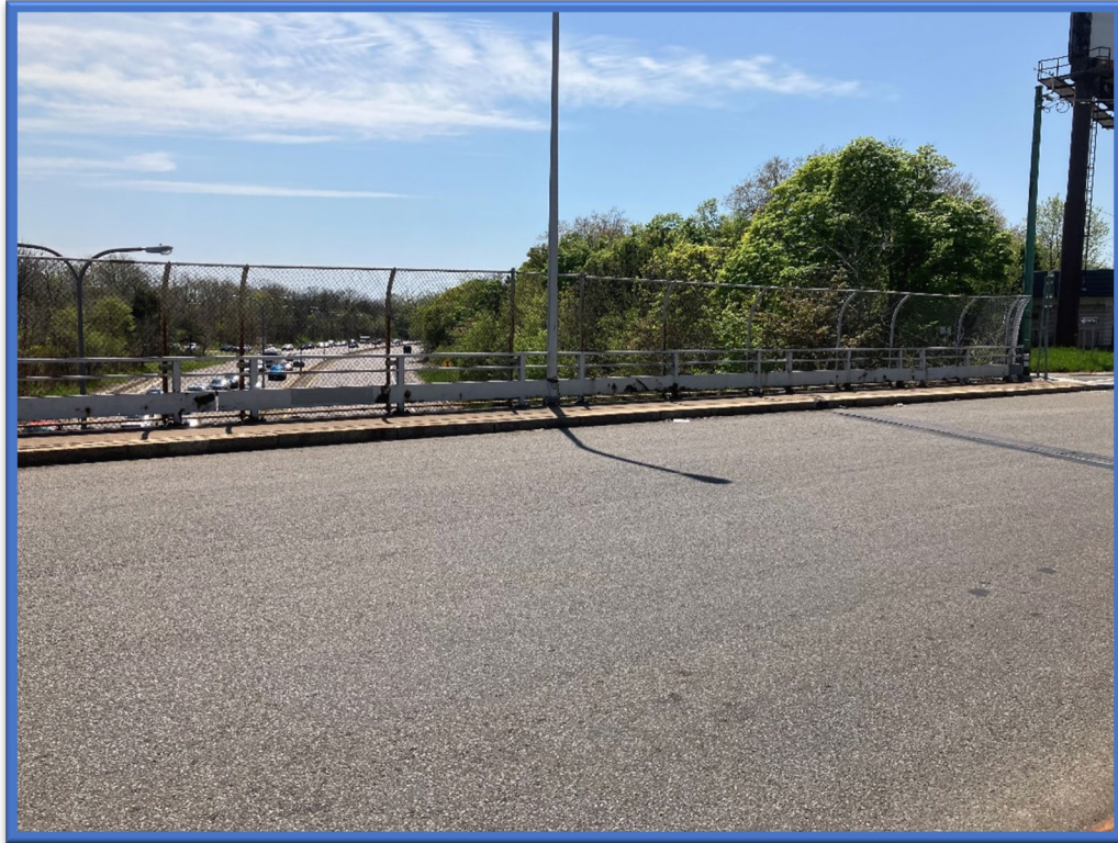
Photo 3 - View to the south from the middle of the E Utica St Bridge over Kensington Expressway (Route 33) (BIN 1022630).
