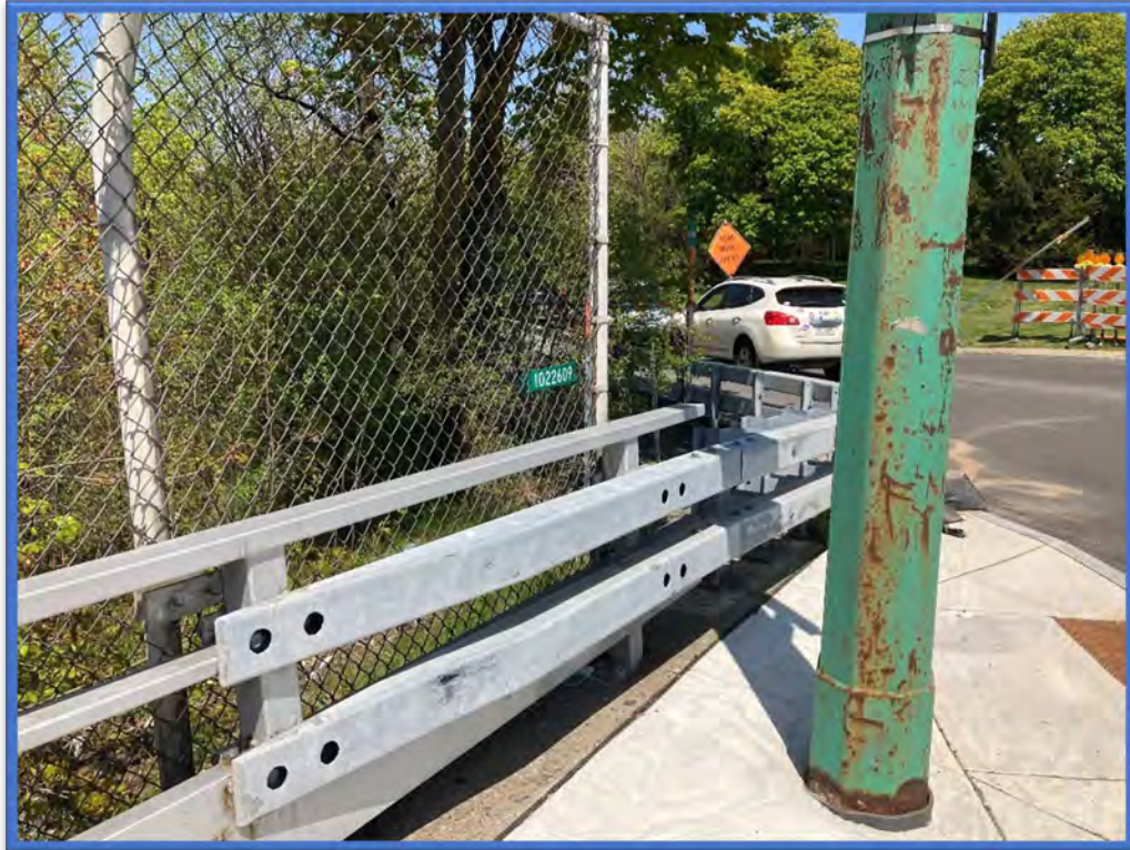
Photo 5 – BIN plate located on the adjacent fence at the northeast quadrant of BIN 1022609.
