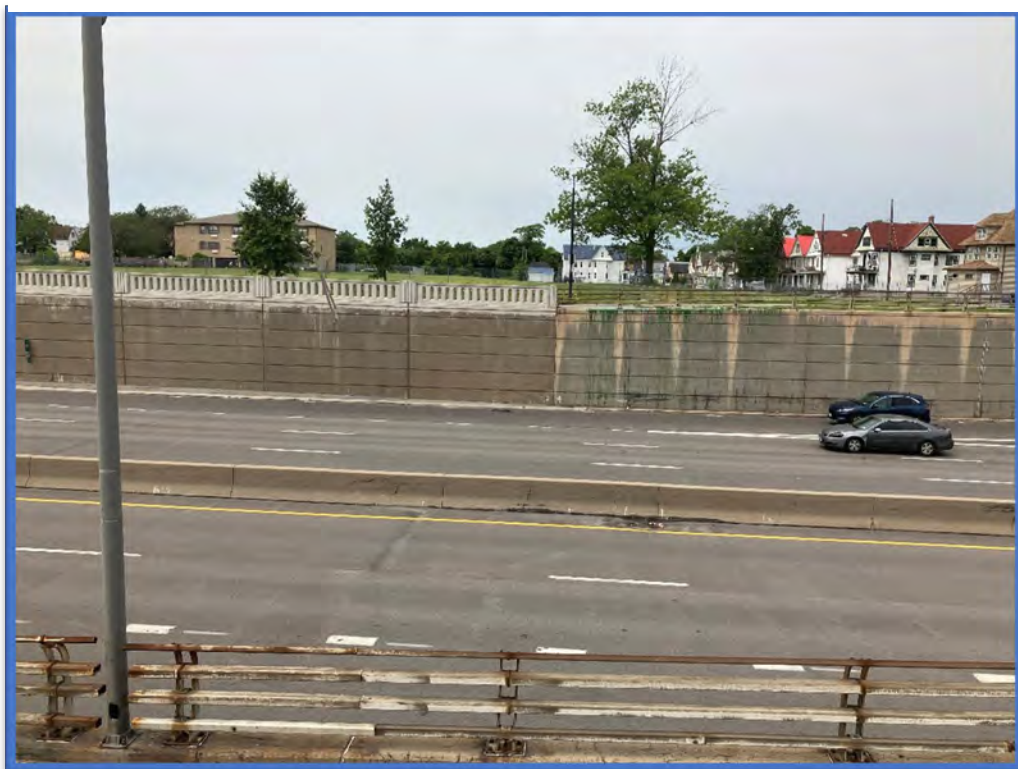
Photo 8 - Asbestos-containing railing post base caulk is associated with all of the metal guiderails located on top of the northern retaining walls. No asbestos-containing caulk is associated with the new decorative concrete guide rails located on top of the southern retaining walls.
