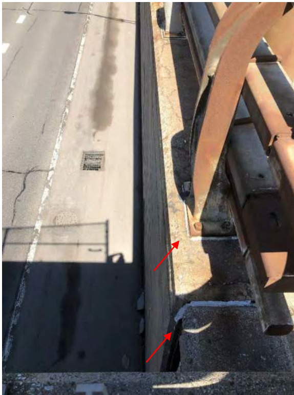
Photo 8 – View facing north at the northeast corner of BIN 1022630 and the retaining wall. The retaining wall grey caulk and the retaining wall guide rail post base grey caulk have both been identified as an ACM.
