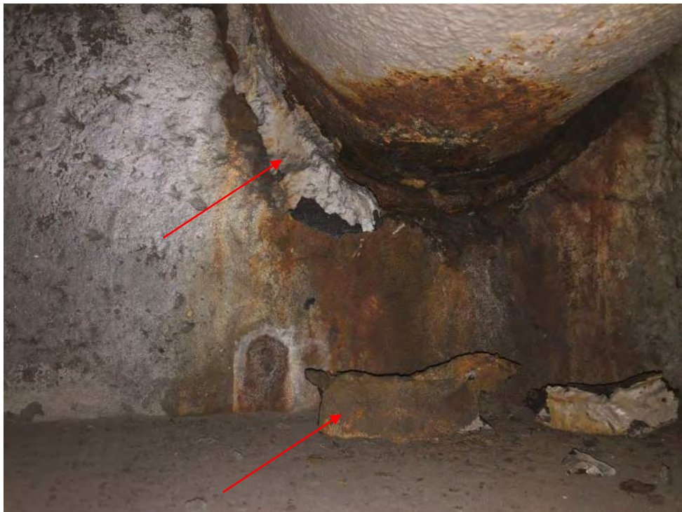
Photo 6 – View of the degraded asbestos-containing packing/sealant associated with the gas utility conduit at the west abutment of BIN 1022630.
