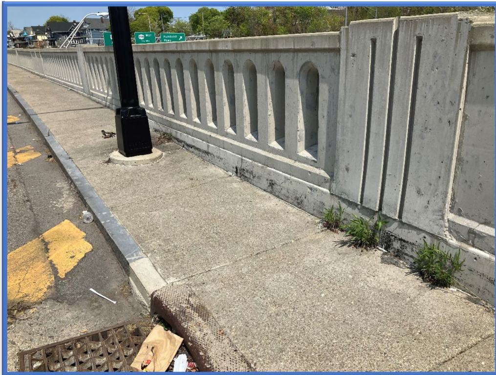
Photo 6 – View of the recently installed decorative upper portion retaining wall adjacent to BIN 1022620. Additional suspect ACM was identified and sampled, however all samples associated with the upper portion were negative for asbestos. The ACM caulking is only associated with the older lower portions of the retaining walls system in this area. (See Photos 4 & 5)
