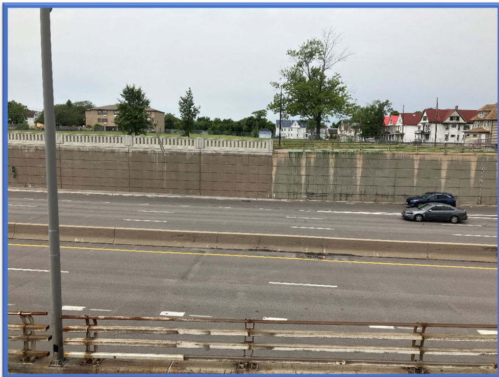
Photo 8 - Asbestos-containing railing post base caulk is associated with all of the metal guidrails located on top of the northern retaining walls. No asbestos-containing caulk is associated with the new decorative concrete guide rails located on top of the southern retaining walls.
