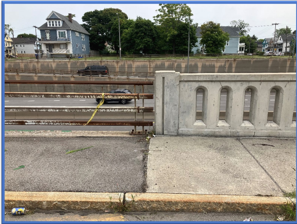
Photo 7 - Asbestos-containing railing post base caulk is associated with all of the metal guidrails located on top of the northern retaining walls. No asbestos-containing caulk is associated with the new decorative concrete guide rails located on top of the southern retaining walls.
