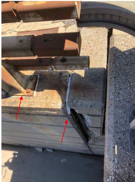
Photo 7 – View facing east at the northeast corner of BIN 1022630 and the retaining wall. The retaining wall grey caulk and the retaining wall guide rail post base grey caulk have both been identified as an ACM. The retaining wall caulk is degraded in places.
