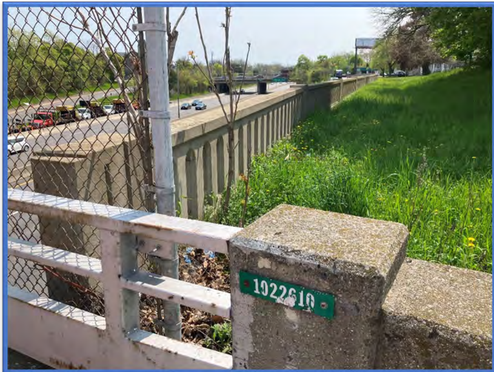
Photo 4 - View of the BIN plate located on the southwestern corner of the Dodge Street Bridge over Kensington Expressway (Route 33) (BIN 1022610).
