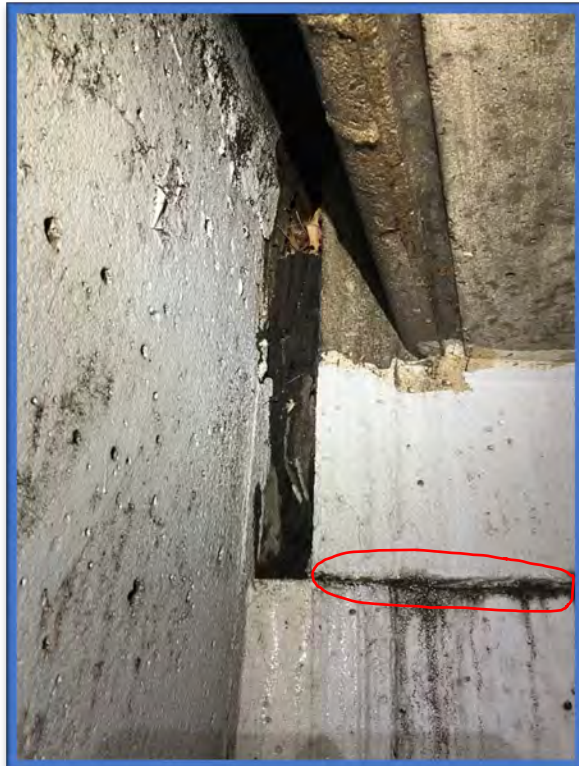
Photo 8 – Compressed asbestos sheet packing located on the abutment shelf at the bridge was previously confirmed as an ACM and visually observed during this inspection of the Dodge Street Bridge over Kensington Expressway (Route 33) (BIN 1022610).
