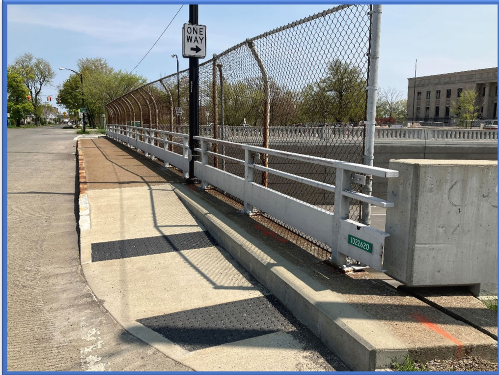
Photo 5 – BIN plate located on the adjacent fence at the southwest quadrant of BIN 1022620. ACM caulking is only associated with the older lower portion of the walls.
