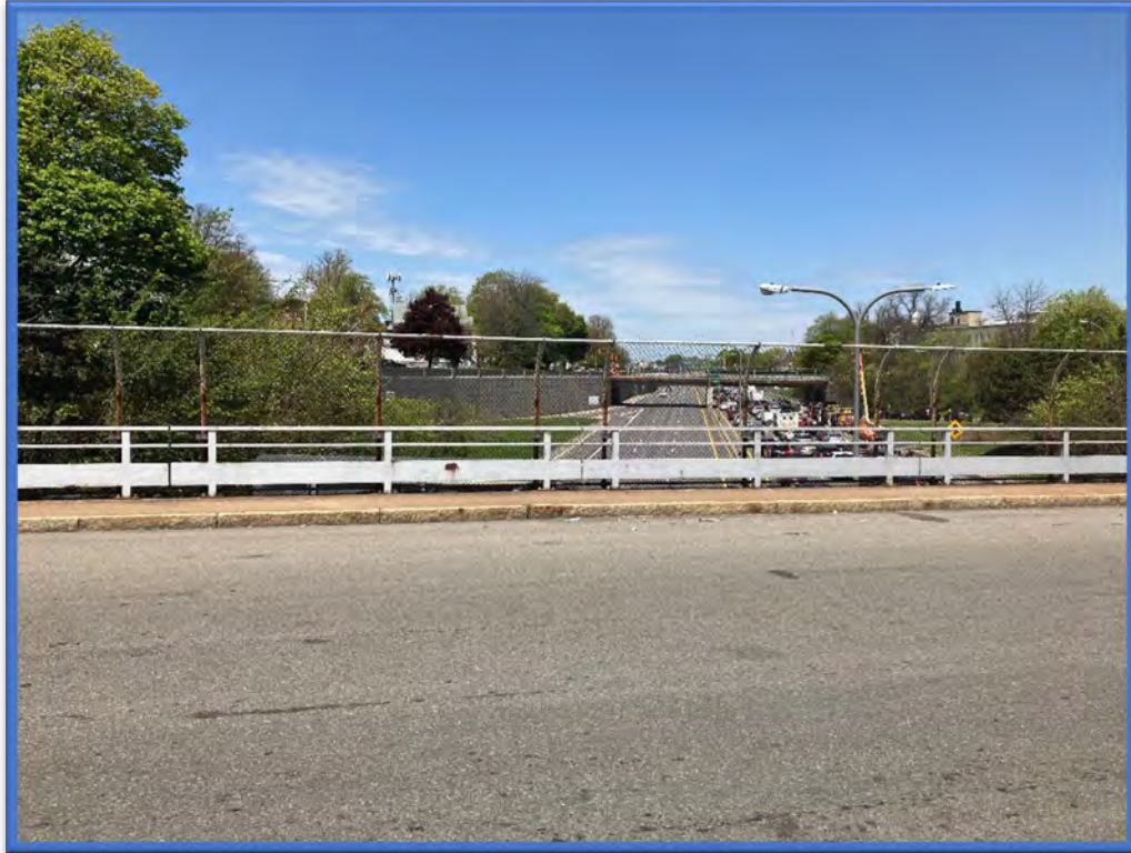
Photo 1 - View to the north from the middle of the Best Street Bridge over Kensington Expressway (Route 33) (BIN 1022609).
