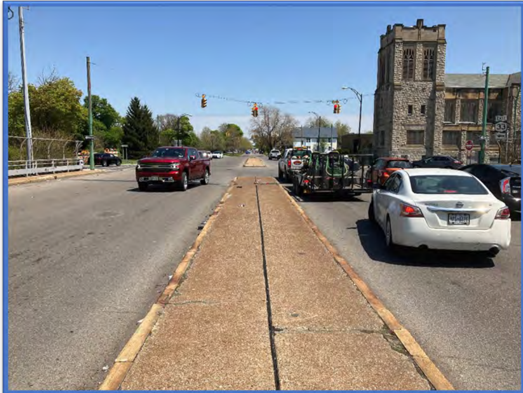
Photo 2 - View to the east from the middle of the Best Street Bridge over Kensington Expressway (Route 33) (BIN 1022609).
