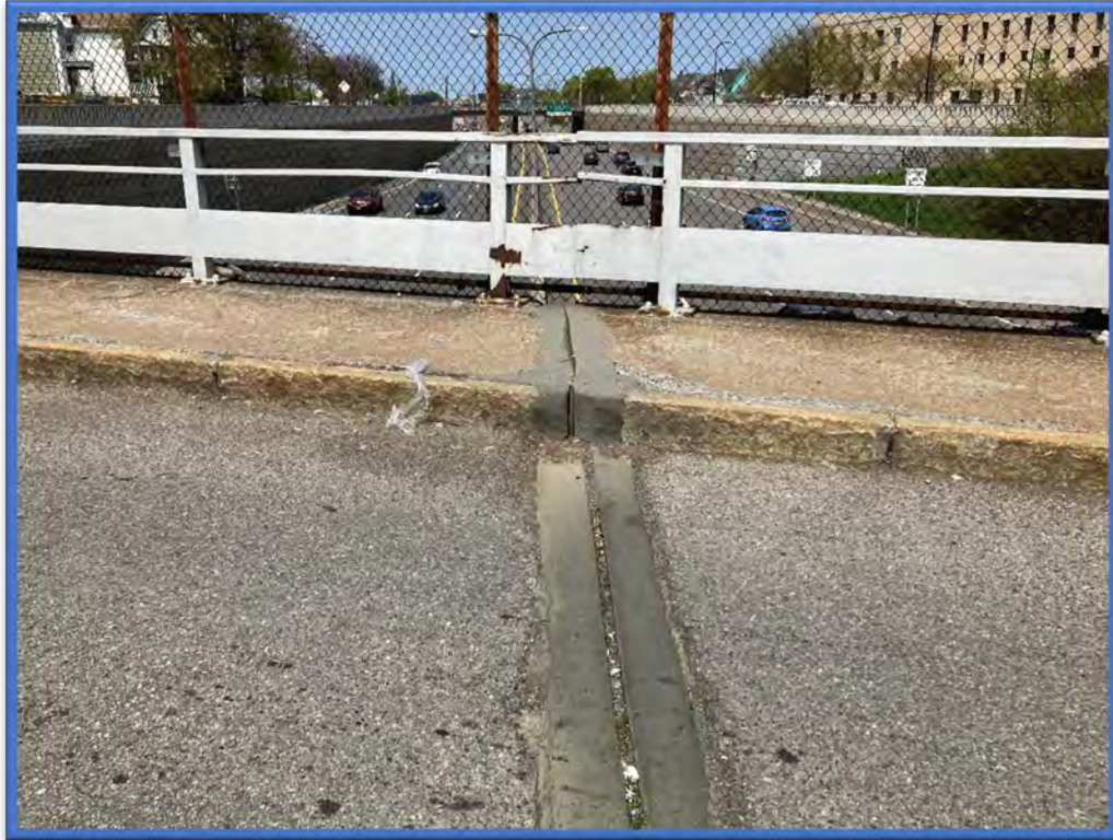
Photo 3 - View to the north from the middle of the Dodge Street Bridge over Kensington Expressway (Route 33) (BIN 1022610).
