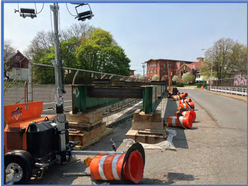
Photo 2 - View to the northwest of the southern side Dodge Street Bridge over Kensington Expressway (Route 33) (BIN 1022610). Repairs to the structure were being conducted at the time.
