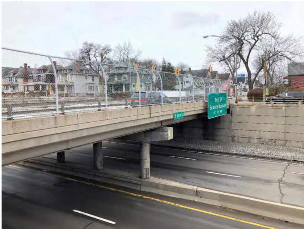
Photo 1 – View looking east at BIN 1022630 (E. Utica Street over Kensington Expressway (NY Route 33)).
