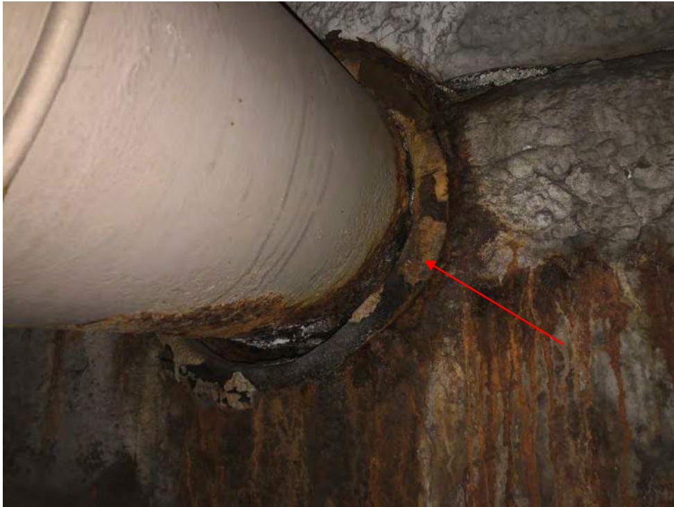
Photo 5 – View of the 12” metal conduit associated with the 8” gas utility line where it penetrates the east abutment of BIN 1022630. The packing/sealant around the perimeter of the 12” conduit where it penetrates each abutment has been identified as an ACM.
