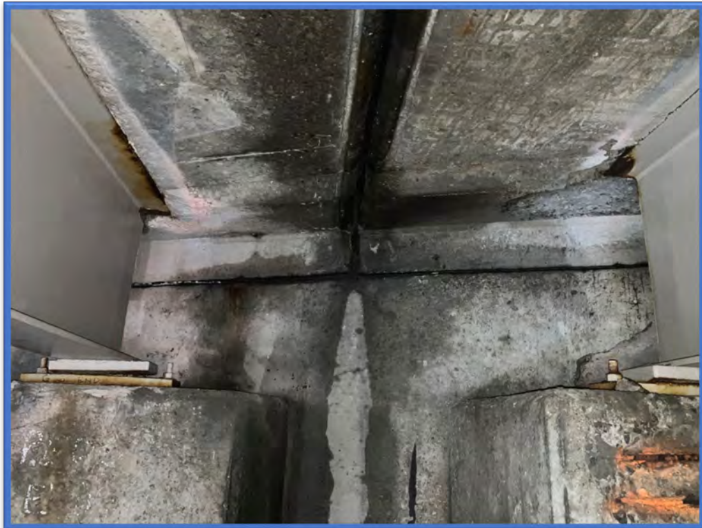
Photo 8 - Compressed asbestos sheet packing located on the abutment shelves at BIN 1022609 was confirmed as an ACM. Picture taken at the center of the east abutment.
