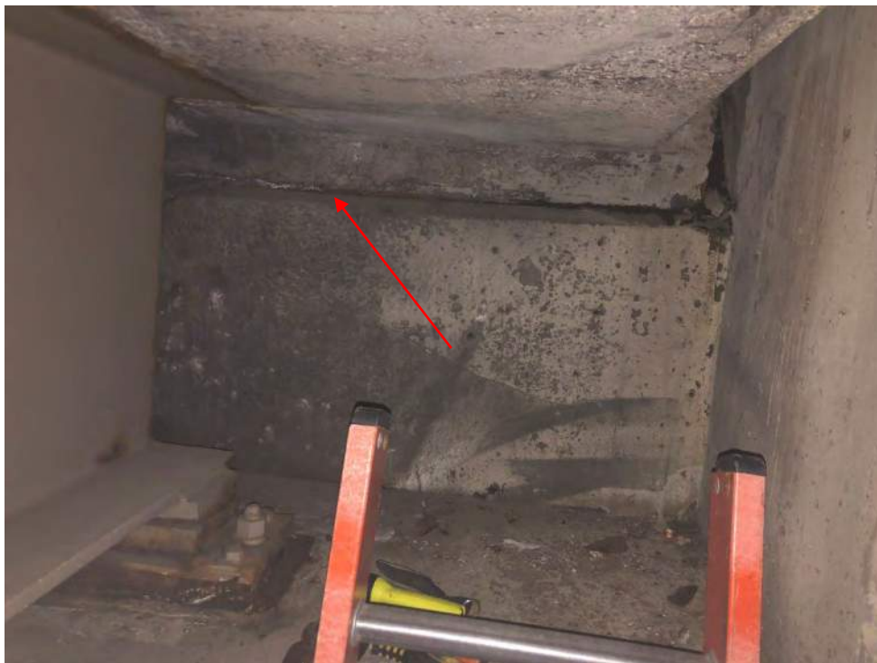
Photo 4 – View of the grey sheet packing that has been identified as an ACM at BIN 1022630.
