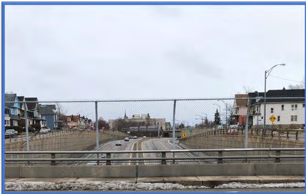
Photo 10 - Retaining wall system within the Kensington Expressway project corridor that has an associated asbestos-containing caulking located within each expansion joint and an inaccessible/assumed asbestos-containing waterproofing located on the back sides of the abutments, retaining walls, counterforts, and tops of footer piles.
