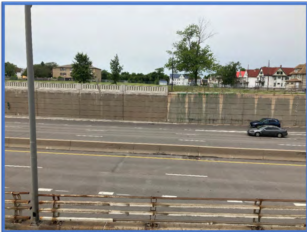
Photo 12 - Asbestos-containing railing post base caulk is associated with all of the metal guiderails located on top of the northern retaining walls. No asbestos-containing caulk is associated with the new decorative concrete guide rails located on top of the southern retaining walls.
